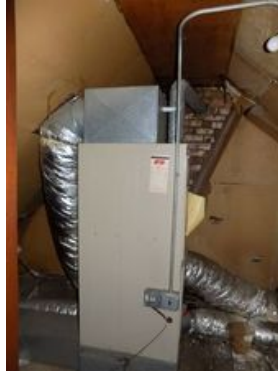
Utility Room-2nd Floor
